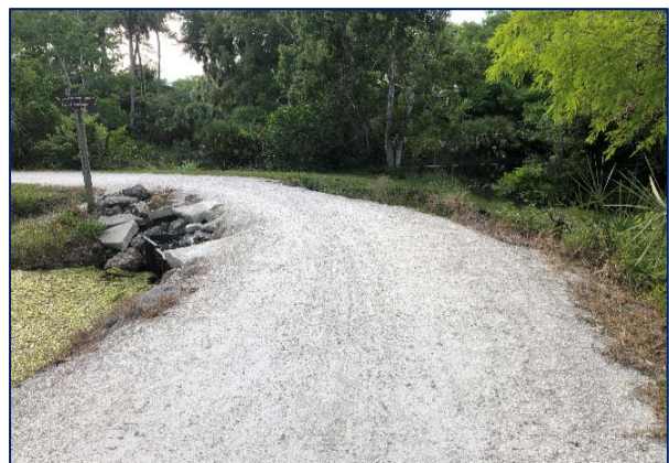
Riverbend Park, Jupiter Damaged Pathway and Culvert
